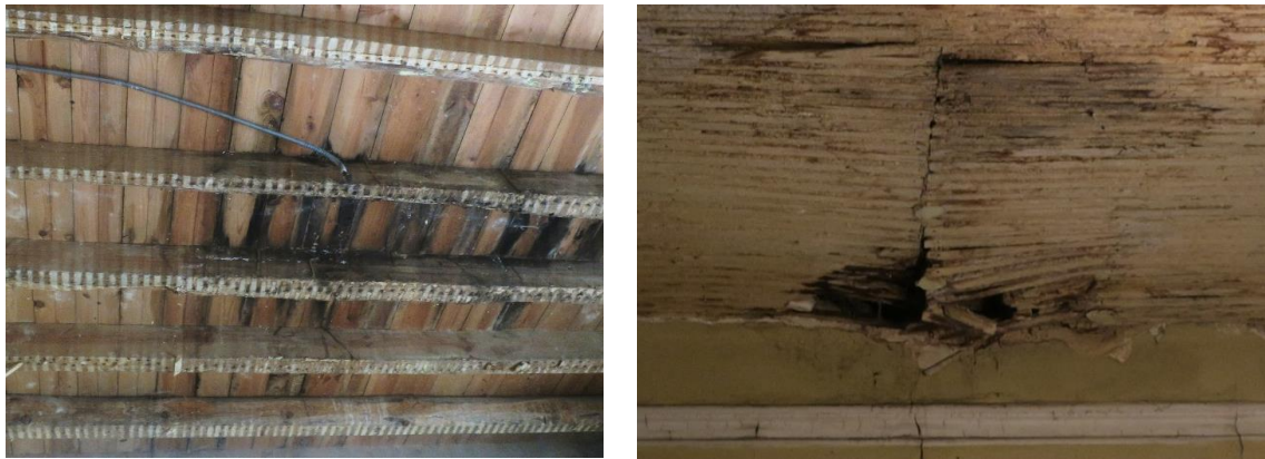
Figure 4.1 - Photographs of timber pavements degradation state in Rua da Esperança do Cardal
